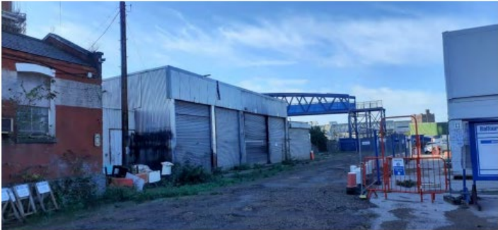
Image 2: View west towards existing storage units and the new footbridge from within the Balfour Beatty site. The site office is on the right hand side of the frame.
